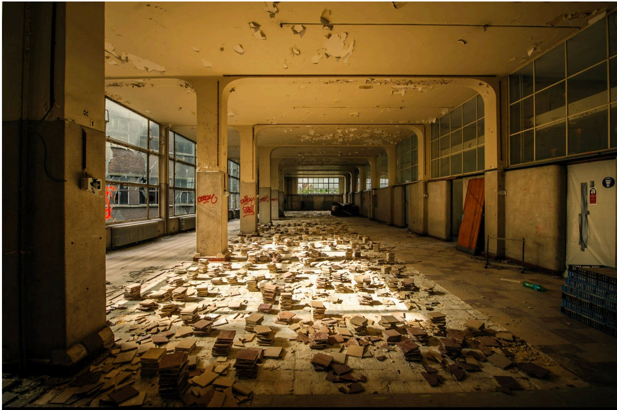
Floor and wall tile reclamation by Rotor DC, the materials reuse spinoff of cooperative design practice Rotor, Brussels, Belgium. Ophoto, 2020
