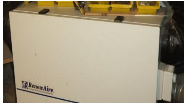
Figure 12 ERV system in Basement
