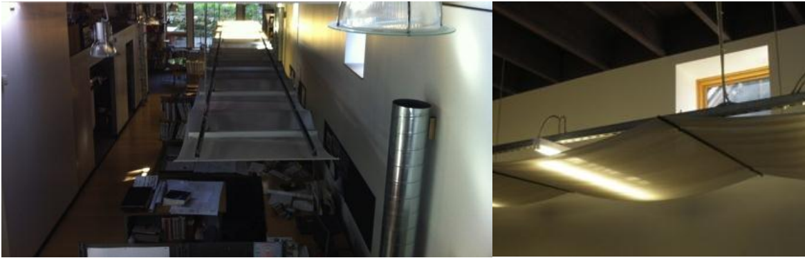
Figure 32 Lighting fixtures and softner(fabric screen)
