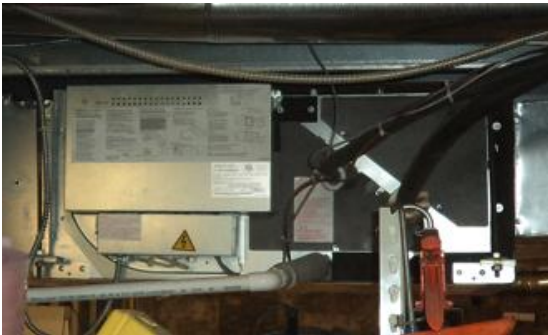
Figure 11 Bryant FE4A Air Heat Pump
